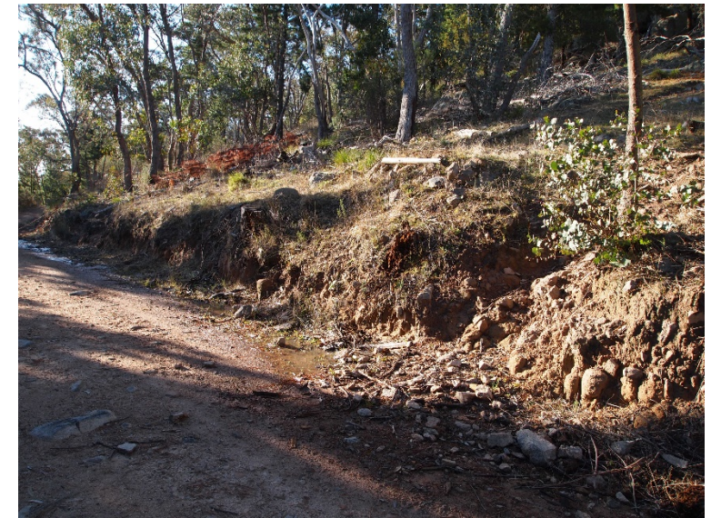
Plate 2: View of one of the road gap jumps.
